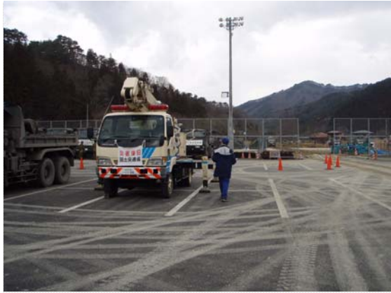
仮設浴場照明車 (3/23)
